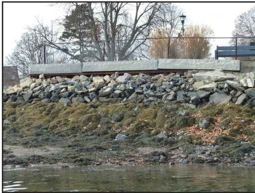
9. Adjacent to T-Head pier Steel sheeting with granite coping and placed rip rap armoring.
