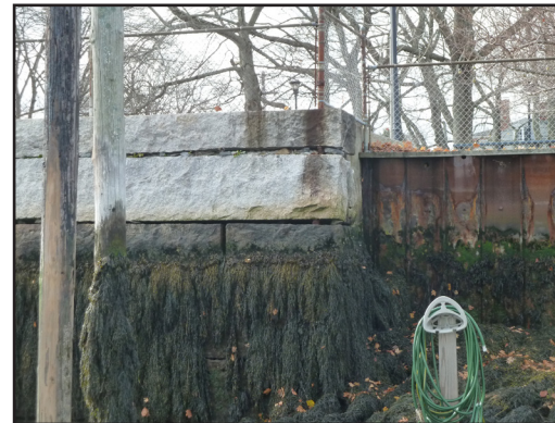
18. From quaywall to steel bulkhead Transition to steel sheeting. Estimated age 20 years.
