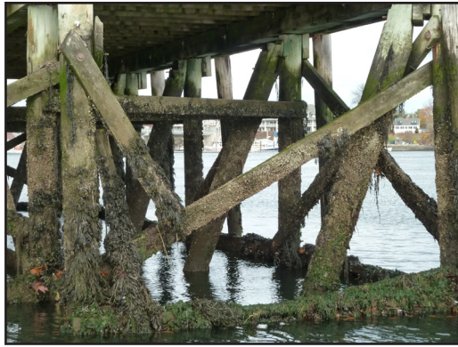
7. South pier Broken cross members under deck, it is recommended to replace the failed bracing member as soon as possible. The structure has 15 years of service life remaining, assuming it is repaired and maintained.
