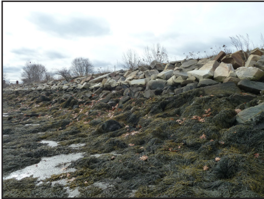
25. Four Tree Island Dumped rip rap along east shore.
